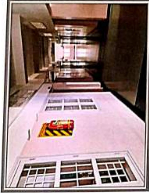
View of Corridor & Fire Extinguisher
